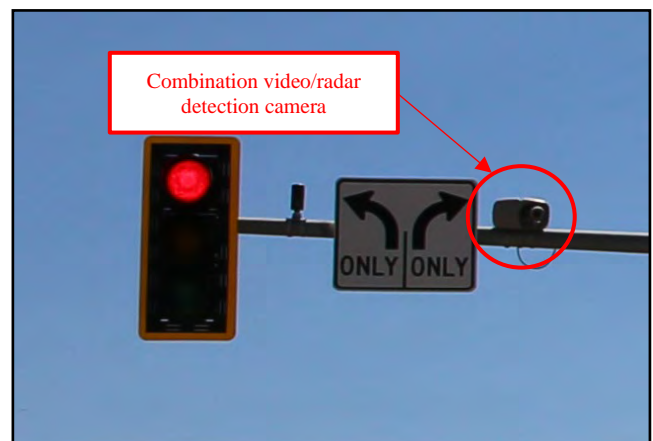
Figure 4. Combination video/radar detection camera facing Roberts Street in the south direction.
